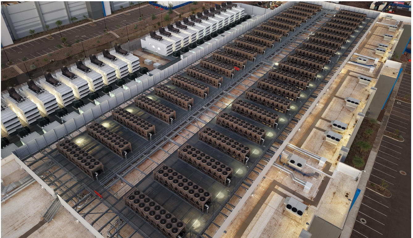
Roof of a data center showing cooling equipment and backup generators. These systems support temperature control and power continuity for high-density computing operations by managing heat and providing on-site electricity during outages. Photo by Rspark3 (Wikimedia Commons).
