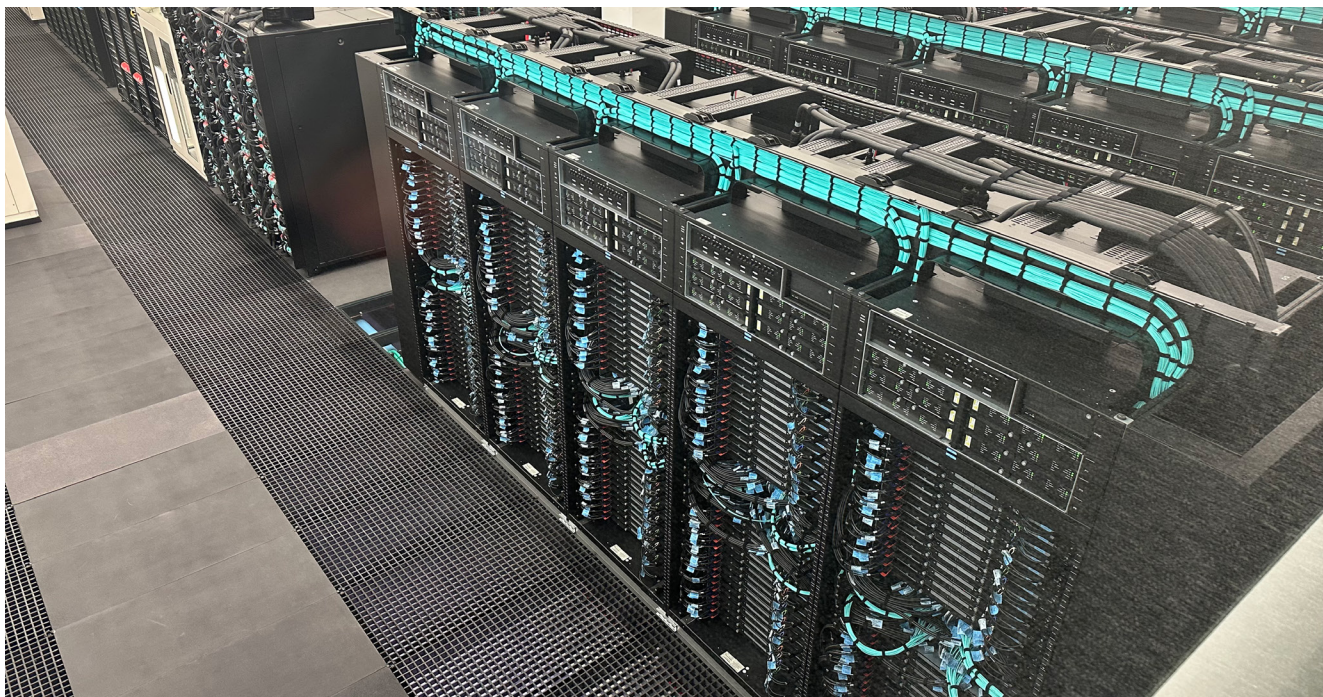
An interior view of MareNostrum 5, a flagship European supercomputer, inside the historic chapel at the Barcelona Supercomputing Center in Spain. The system is among Europe's most powerful high-performance computing installations, delivering around 314 petaflops of computing power. It is currently being upgraded under the EuroHPC Joint Undertaking's BSC AI Factory initiative to expand Europe's AI capacity, with next-generation GPUs, expanded storage, and energy-efficient cooling to support large-scale AI training and advanced machine learning for startups, researchers, and public institutions across Europe. Photo by Steve Jurvetson (Flickr).
