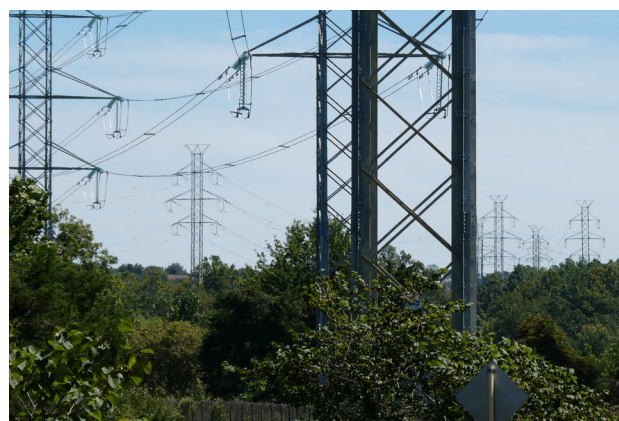
Power transmission lines along the W&OD corridor in Ashburn, Virginia, carrying electricity toward one of the world’s largest concentrations of cloud and AI data centers. Source: Photo by Kit Case (Flickr).
