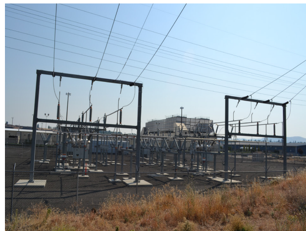
Google Data Center, The Dalles, Oregon, USA — High-voltage transmission lines feed directly into on-site substations, converting grid power to the stable, continuous electricity required to run thousands of servers. Photo by Visitor7 (Wikimedia Commons).
